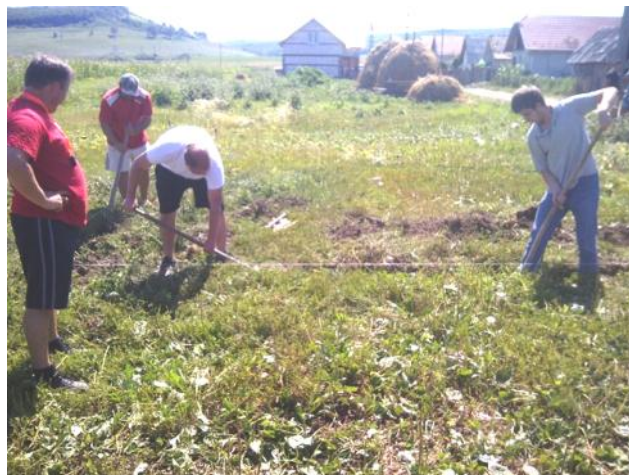
Attila Toth, members of the Gornesti Church and the Leesburg Community Church team begin preparing the site of the new Gypsy Mission Center by marking guides for the foundation and framing.
