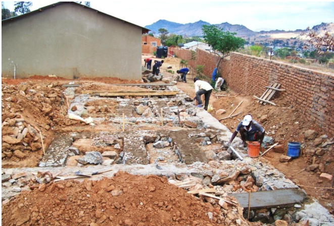
Work on the foundation of the new dormitory at Daily Bread Life Children's Home began in October.
