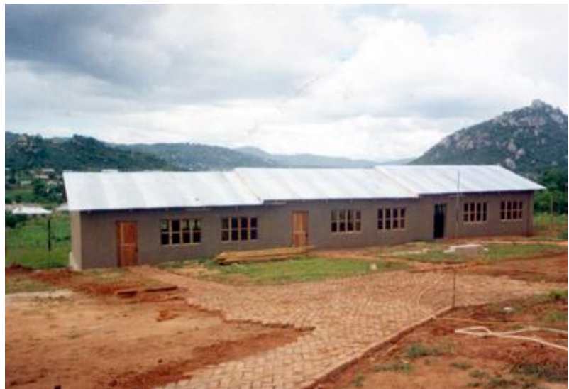
With the installation of the roof, doors and windows and the walkways laid, the orphanage is ready for the children.
