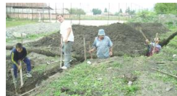
Attila Toth, second from left, and others work on renovating the property for a new church in Gernyeszeg, Romania.
