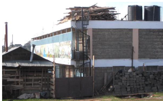
Included in the final construction phase was the adding of a second floor, a spiral fire escape, and water storage tanks.
