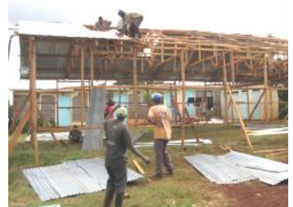
A temporary structure for worship services and church activities is built while the new facility is under construction.
