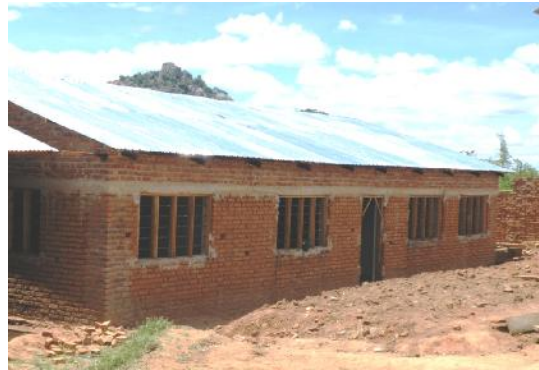
Construction of a new dormitory at the Daily Bread Life Children's Home began last fall and upon completion will house children there who have reached secondary school age.
